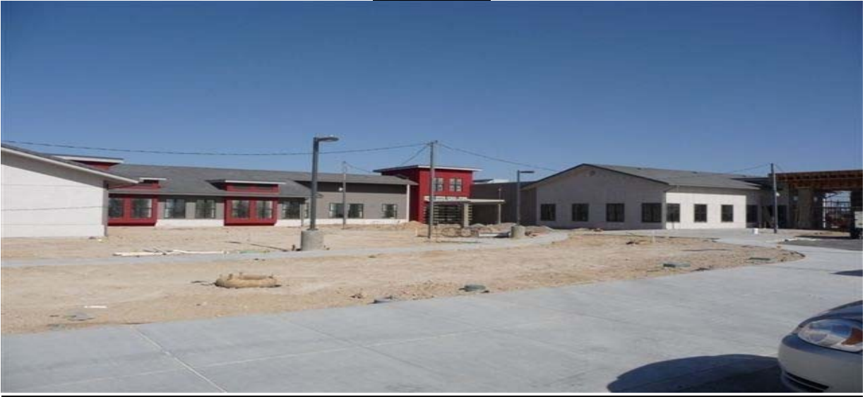
The William J. “Pete” Knight Veterans Home of California—Lancaster (under construction, May 2009).
